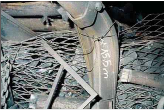
Obr. 2 Detail deformace průřezu TH 29 [3] Fig. 2 Detail of TH 29 cross-section deformation [3]
